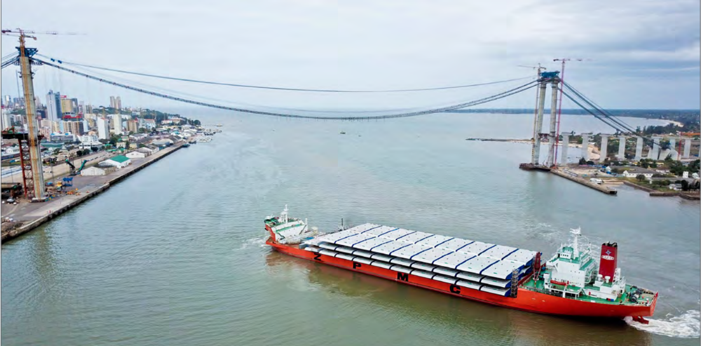
The 57 massive box girders for the main span arriving from China on 27 September 2017 (the main span across the bay will have a clearance of 60 m, allowing the largest of ships to pass under)
