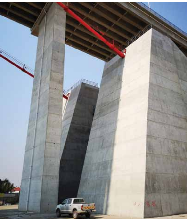
Heat of hydration had to be controlled during the casting of anchor blocks and other elements.
